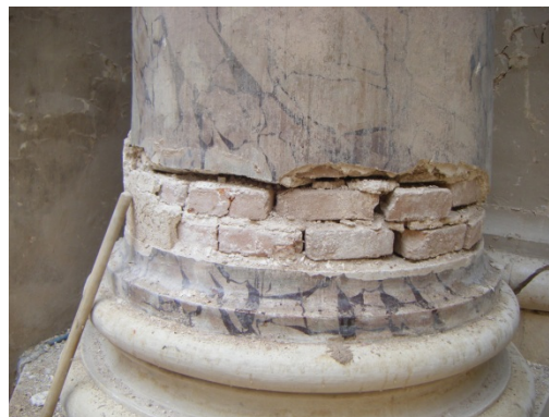
Figure 2.32 – Local damage concentration due to seismic action, an example of a pillar in L'Aquila Cathedral.
