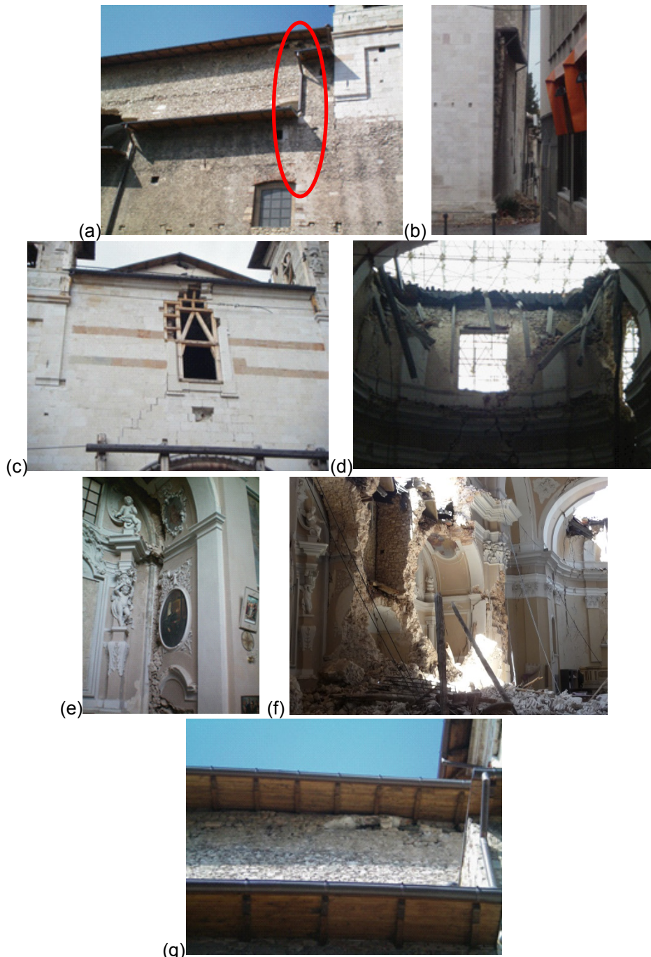
Figure 6.5 - Some mechanisms observed after the earthquake (Silva et al. 2011): (a) overturning of façade and (b) lateral chapel walls, (c) shear mechanism in the façade, (d) collapse of the semi-dome and the roof in the apse, (e) collapse of the lateral chapel and the wall above, (f) disconnection between the chapel wall and external wall and (g) damage under the roof in the south nave wall.
