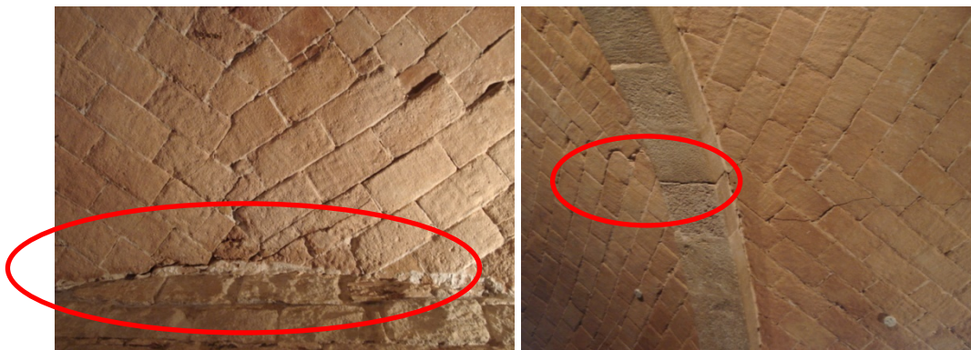
Figure 4.2 – Cracking observed in one of the vaults.
