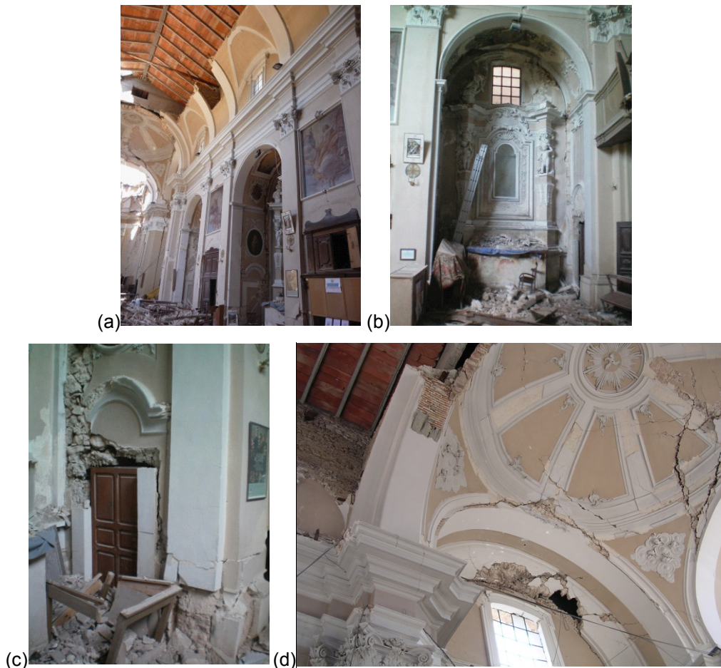
Figure 6.15 - Collapse mechanisms detected by Y direction pushover analysis: (a) arches in the nave, (b-c) walls and buttresses in lateral chapels, d) transept arches.
