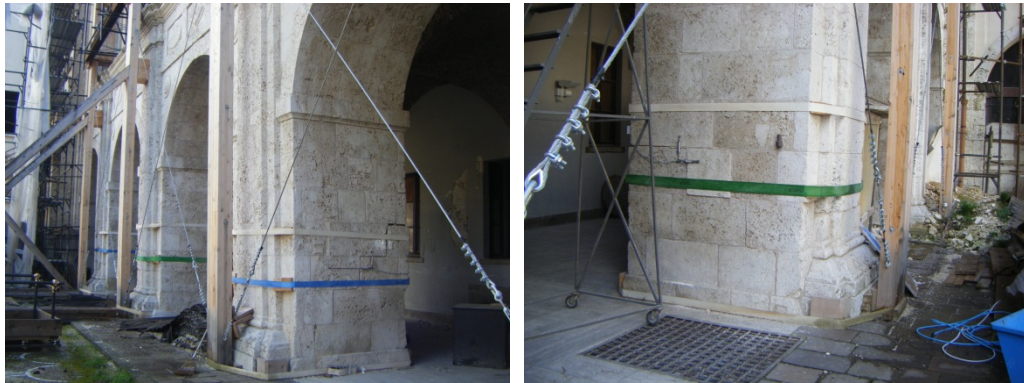
Figure 2.33 – Seismic damaged pillars with emergency measurement in the courtyard of the Spanish fortress in L'Aquila.
