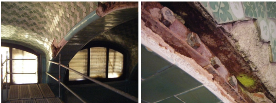
Figure 5.4 – Corrosion of steel profiles embedded in masonry vaults before the restoration works.
