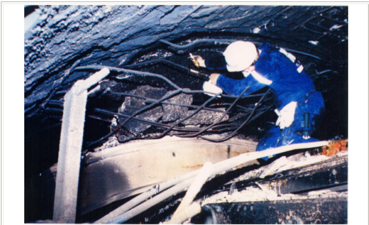
Figure 2-1. Damage of concrete and reinforcement after the Great Belt fire [3].
