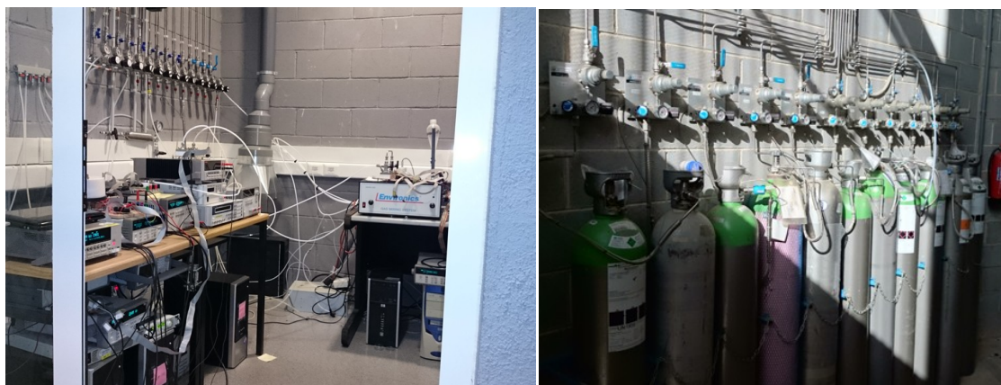
Figure 5.24. (Left) Photograph of the gas measurement room. (Right) Photograph of the basement where the canisters are located
