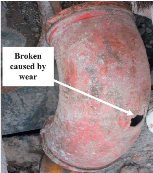
Figure 6.11: The destroyed pipe.
