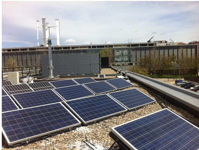
Figure A.7: PV modules in the roof of the laboratory.
