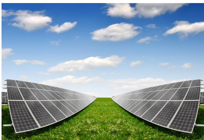
Figure 1.3: PV panels for large surface areas.
