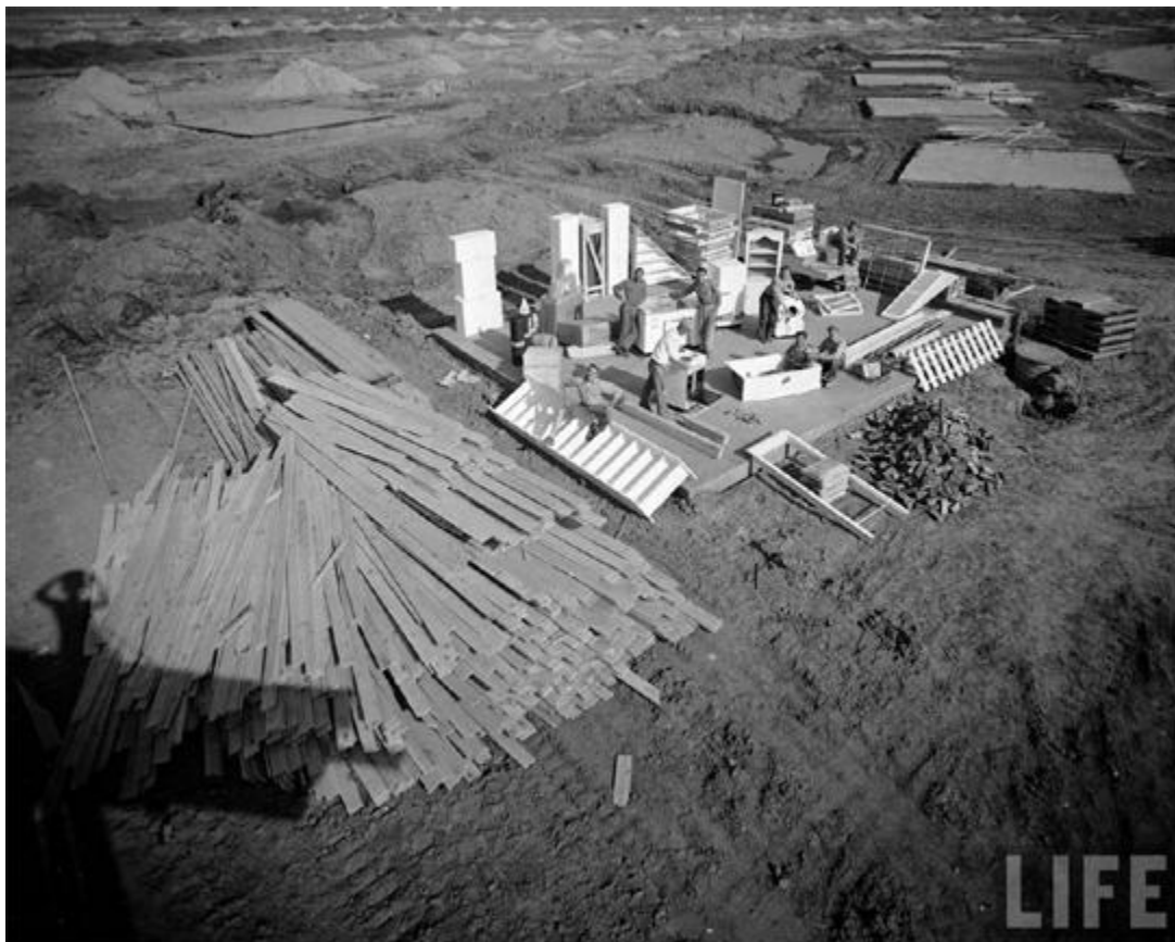
Tony Linck, para Life Magazine , Workmen and the materials to construct a house gathered in a lot before construction , junio, 1948 http://tiger.uic.edu/~pbhales/Levittown/building.html
