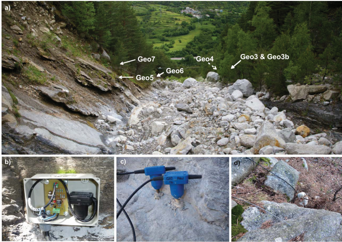
Figure 30: a) Downstream view from inside the channel indicating the places where the geophones are placed. Pictures of the detailed assemblies are shown in (b) to (d).
