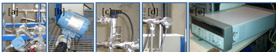
Figure 3.6 - [a] Solution flow meter, [b] water flow meter, [c] Pressure Transmitter, [d] Temperature sensor, and [e] Data logger.
