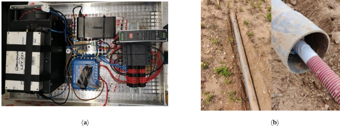
Figure 36. Next-generation NVIS hardware prototypes. (a) Battery-based power supply tested in Hostalric. (b) Underground antenna tested in Cambrils.
