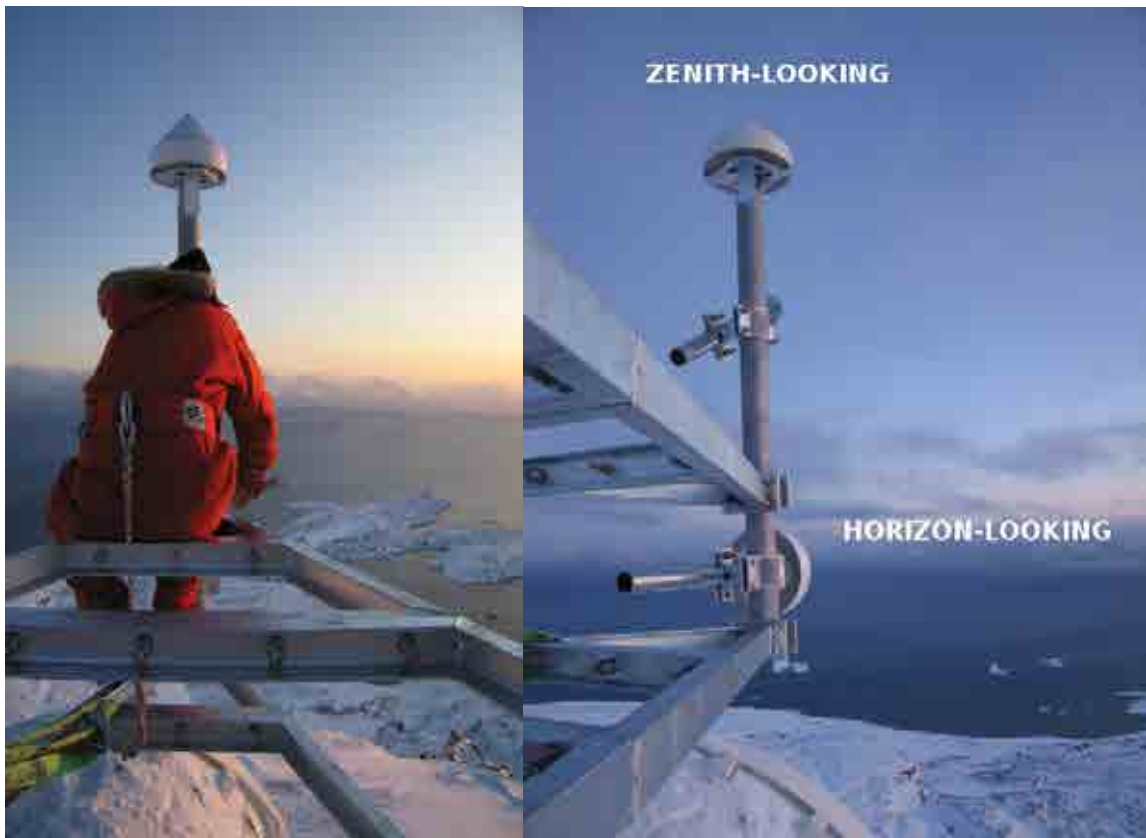
Figure 20.: Images of the antenna system mounted on the telecommunications tower, overlooking Disko Bay. Pictures taken in October 2008, during the installation of the equipment for the sea ice campaign.
