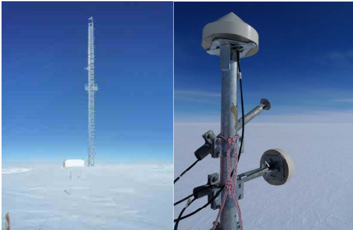
Figure 26.: [Left] American tower, at Dome-c. [Right] Antenna system mounted on top of the American tower, overlooking a protected area of pristine snow. Pictures taken in December 2009, during the installation of the dry snow campaign.
