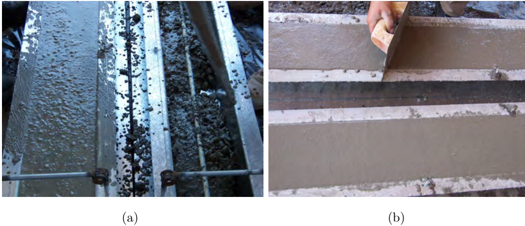
Figure 5.16: Casting sequence; (a) concrete being poured in two layers and (b) compacting and leveling to final surface.
