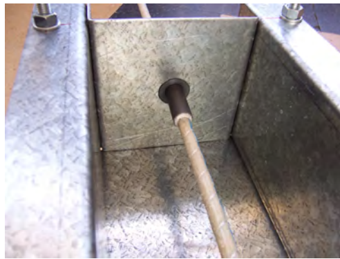
Figure 5.14: Detail of the plastic pipe bond-breaker and aligning annulus when reinforcing rebar already placed in the mould.
