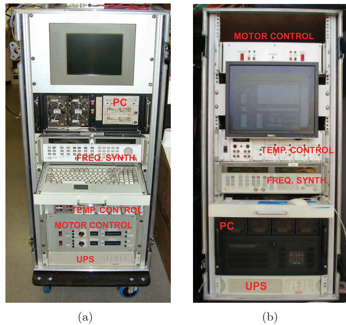
Fig. 4.2: View of the LAURA radiometer control rack, (a) before, and (b) after the update.
