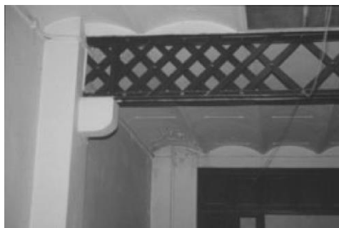
Figure 3.34 - Position of a steel beam at the ground floor and transmission of the load to a masonry column by a simple support (Paricio Casademunt, 2001).
