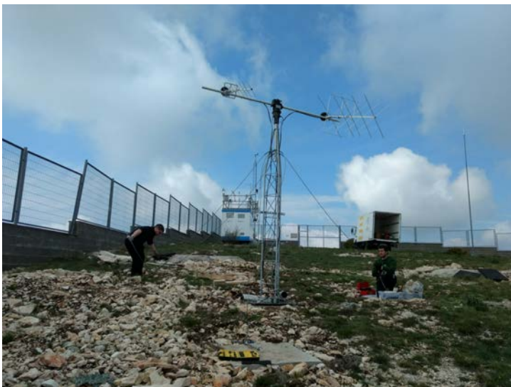
Figure 8.3: VHF/UHF antenna at the UPC/IEEC Montsec Ground Station while it was being installed in 2018.
