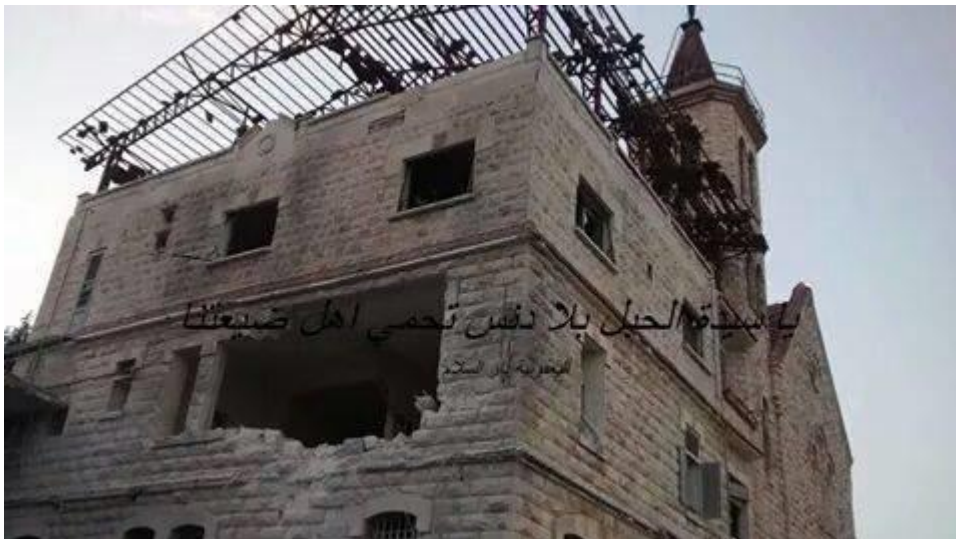
Figure 43- Picture reflecting the damages at the Ya'qubya Church following a government air strike – Source: Facebook Page
