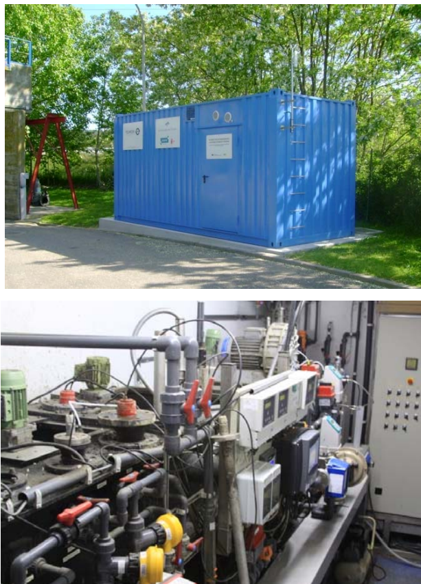
Figure 3-1: The containerised MBR-RO pilot plant, (a) external view, (b) internal view.
