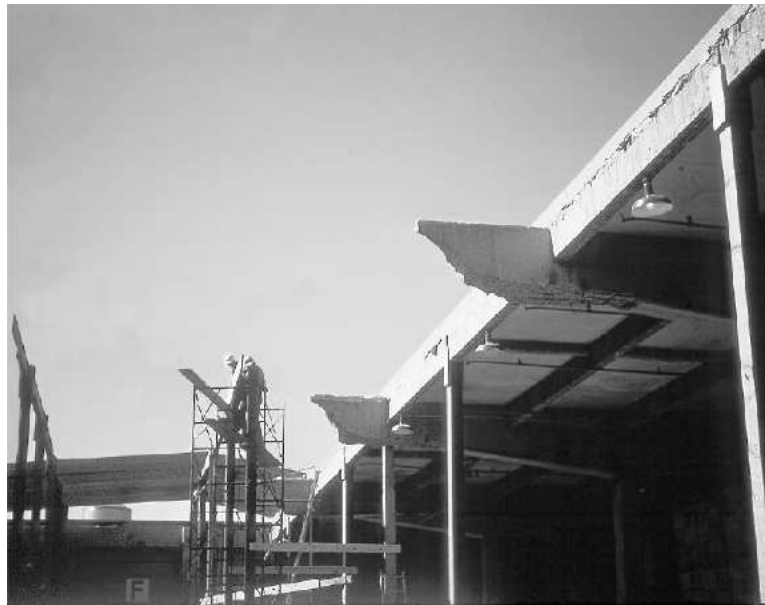
Figure 1.5: American Air Force warehouse shear failure.
