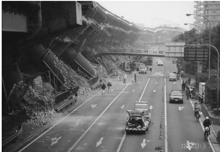
Figure 1.6: Shear failure of Hanshin express piers during Kobe earthquake 1995.
