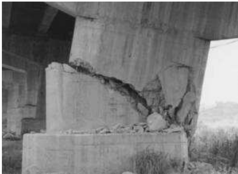
Figure 1.7: Shear failure of squat bridge pier during Taiwan 1999 earthquake.
