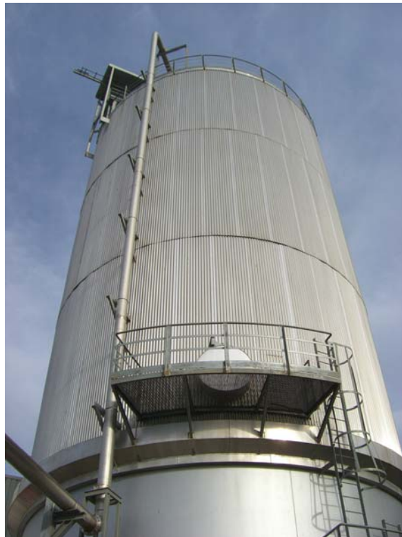
Figure 7.3. Anaerobic digester installed in the plant.
