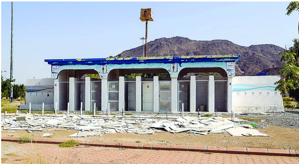
Figure 1.6: Broken doors of one of the toilet complexes
