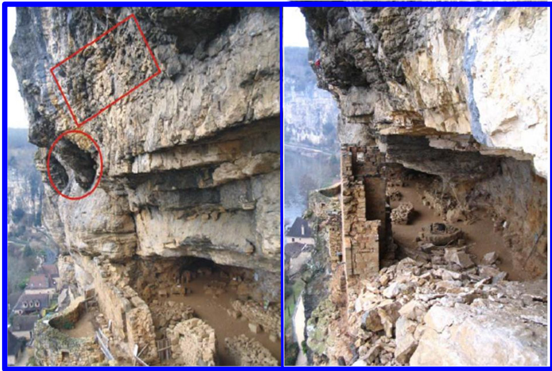
Figure 8.207: (a) Blocks capable of slide and require support, (b) Cavern and masonry wall with loose rock blocks
