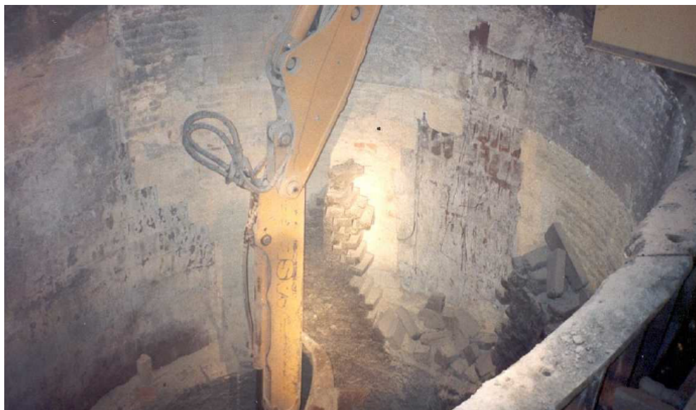
Figure 1.5: Brick wear just prior to removal
